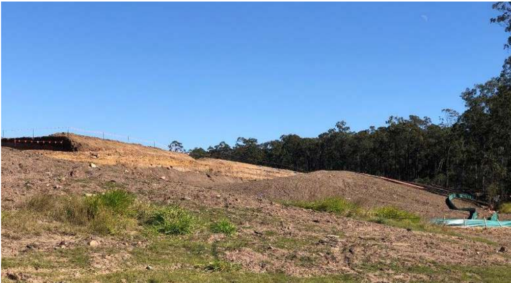
Photo 1: Erosion and sediment control fencing, and fauna friendly fencing on clearing extents post-earthworks.
