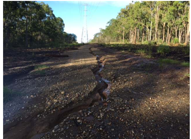
Image 9: Powerline easement through the Goodna Creek open space area and erosion caused by heavy rainfall and flooding from ex-tropical cyclone Debbie
